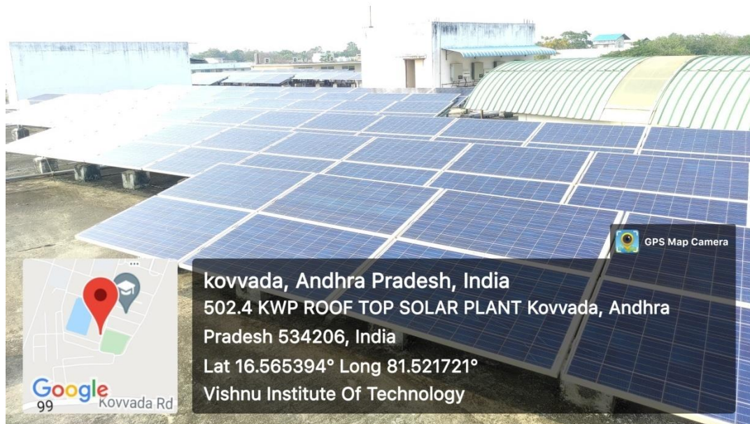
ROOF TOP SOLAR PLANT
